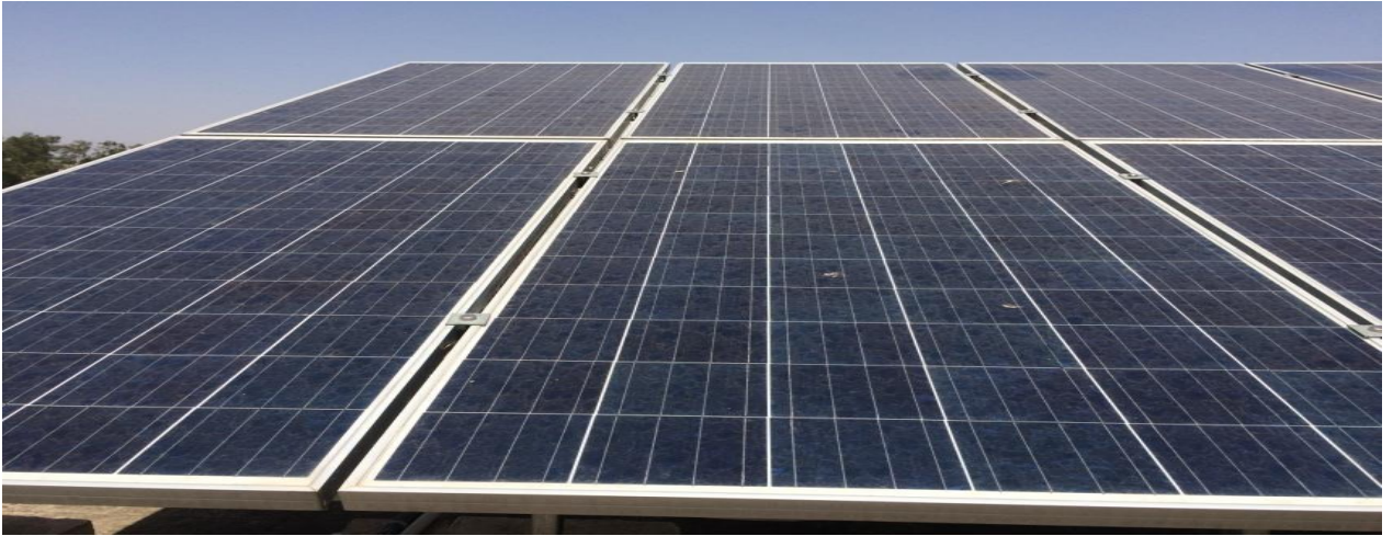
Fig. 1: Picture of the lunar panel containing a multi-crystalline silicon lunar cell that is installed in the CME building.
