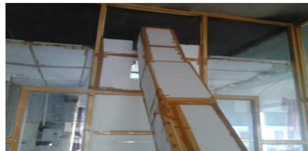
Figure 3 Centrally Duct Arrangement Setup
