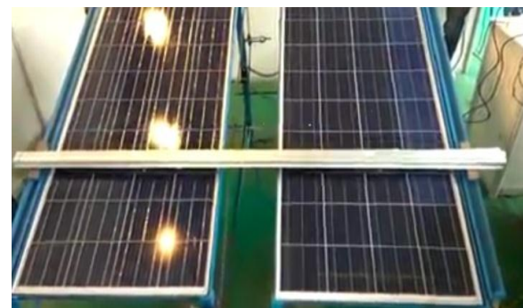
Figure 5 Automated cleaning system
